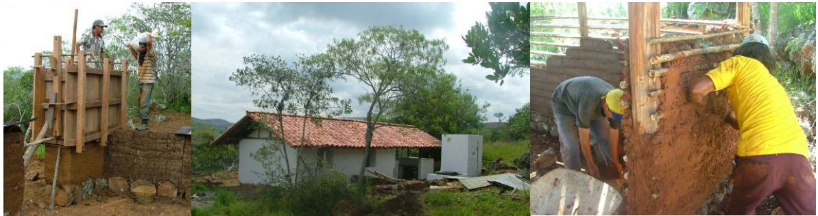
Popular contemporary housing, Barichara-Colombia. Fundación Tierra Viva, Architect: Jesús Antonio Moreno C.
